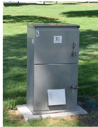
S11. Electrical box
