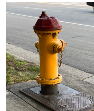
S29. Fire hydrant
